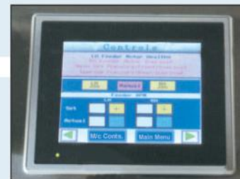
PLC based touch screen controls
